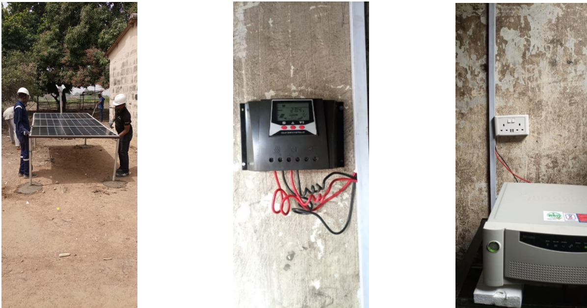
Figure 1 - Installation in Oyo State, Nigeria.
