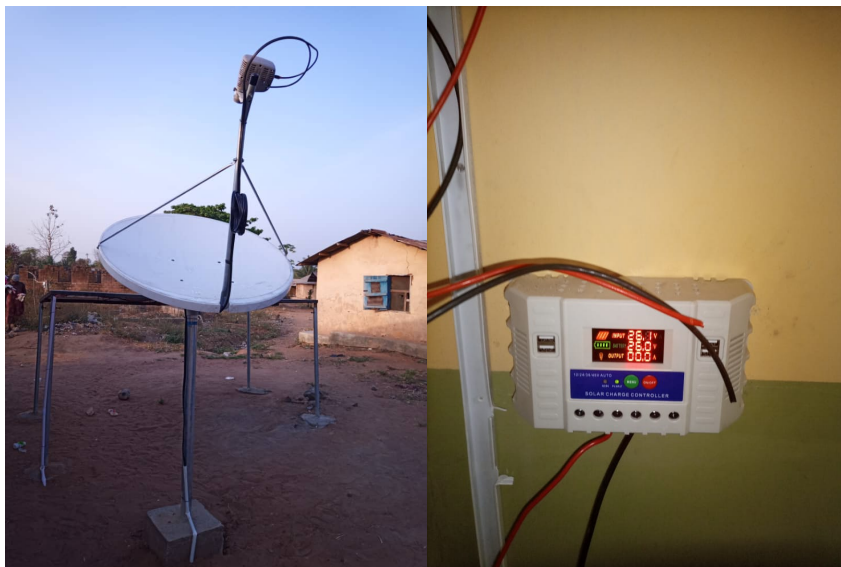
Figure 2 - Installation, Oyo State, Nigeria.
