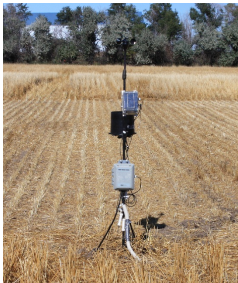
Fig. 1. Cellular Modem with Solar Charger, Data Logger, and Rain Gauge.
