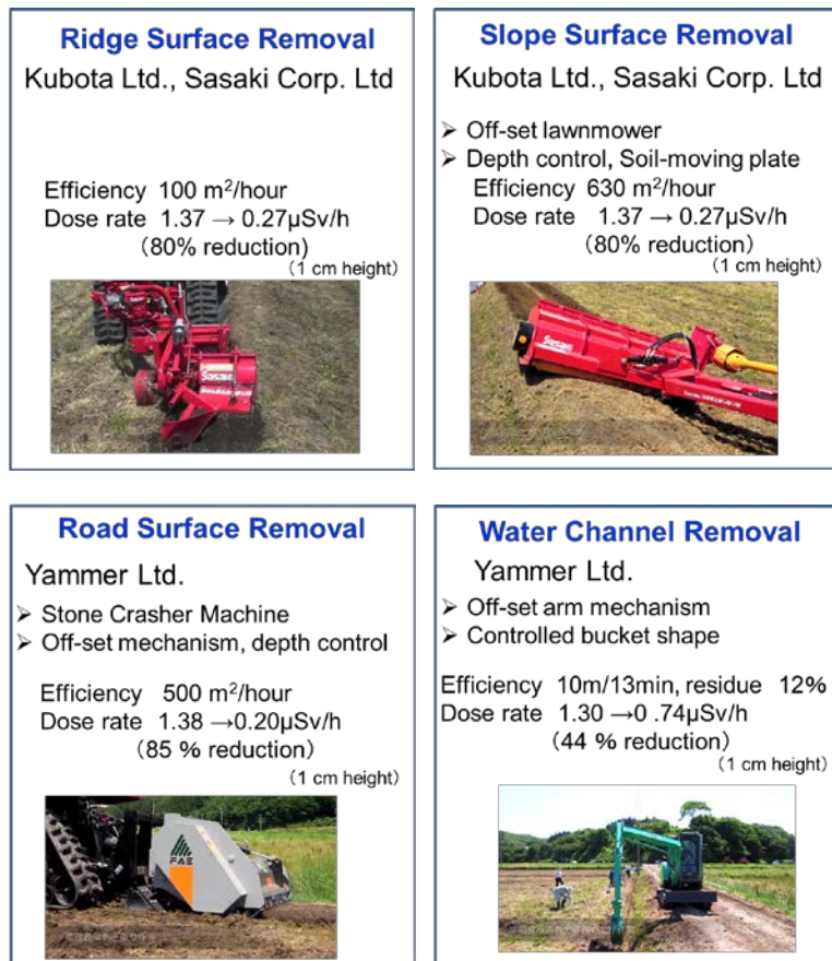
Figure 3. Top soil removal machines to clean off the radioactive materials across the fields.
