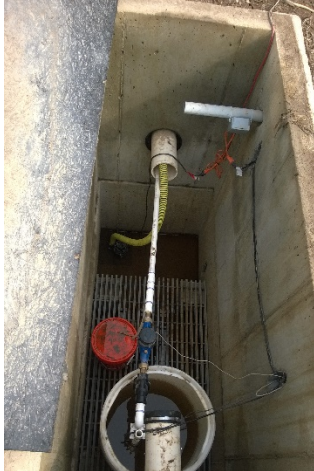
Figure 2. Water flow measurement and sampling installation.
